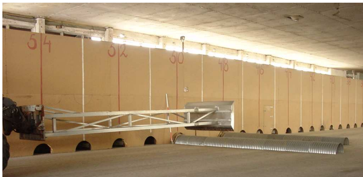
Figure 4.8: Grain storage and ventilation facility used on DE 1300MB
