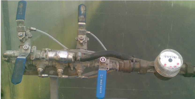
Figure 13: Section shutoff valves and flowmeter
