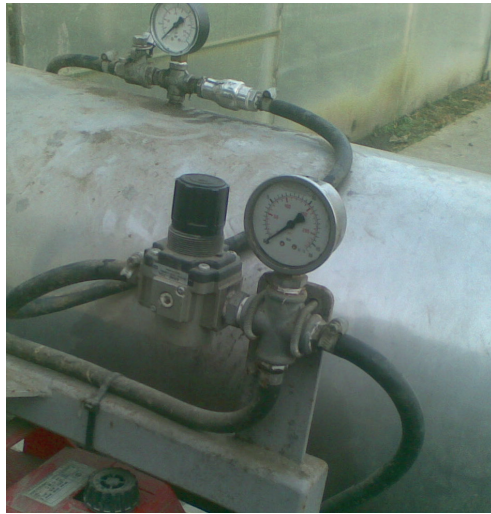
Figure 14: Air pressure adjustment valve.
