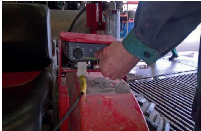
Figure 15: Pump potentiometer controls
