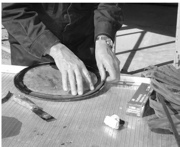
Figure 3 Replacing old worn seals of grain silo hatch to improve fumigation efficacy.
