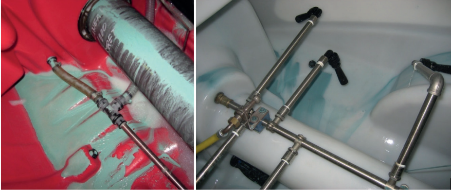
Figure 19. New sprayers shall be provided with a well-designed agitation system
