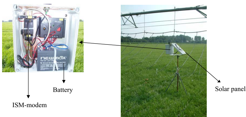
Figure 3.12: Data transmission unit with a solar energy supply
