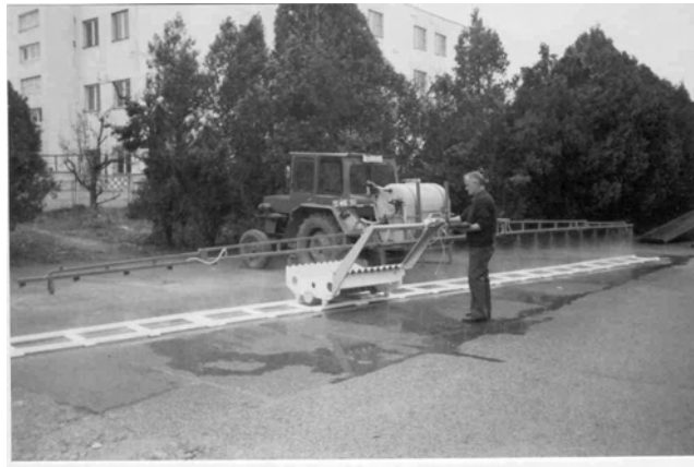
Figure 3 Checking the uniformity of distribution of the EEP 500 equipment with the stand designed by INMA
