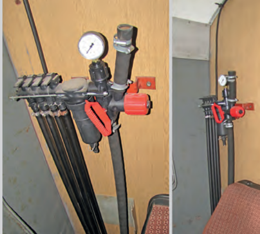
Fig. 6 – Example of manually control of distribution system (photo: A. Godyri).
